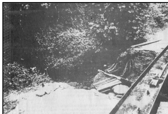
A section of Route 642 in Nottoway County, just south of Crewe, was washed out by heavy rains from Tropical Storm Gaston in August 2004. The steel beam in the photo was placed across the washed-out section of road so vehicles could pass until the road was repaired. (Photo courtesy of The Crewe-Burkeville Journal )
