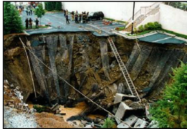
Collapses, such as the sudden formation of sinkholes, may destroy buildings, roads, and utilities. (Photo: Bettmann)
