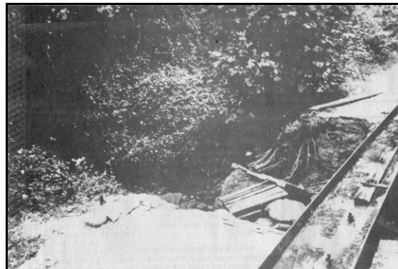
A section of Route 642 in Nottoway County, just south of Crewe, was washed out by heavy rains from Tropical Storm Gaston in August 2004. The steel beam in the photo was placed across the washed out section of road so vehicles could pass until the road was repaired. (Photo courtesy of The Crewe-Burkeville Journal )
