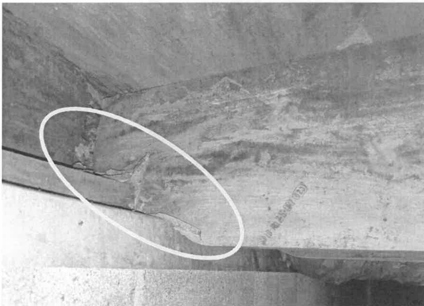
Photo No. 08 Location: Crawl space at western wall. Description: Sill plate and floor joist rotted and crushed.
