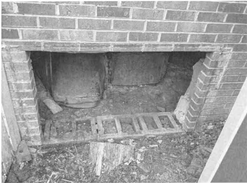
Photo No. 04 Location: Looking south at crawl space entrance. Description: Crawl space entrance general condition, abandoned HVAC ductwork beyond.
