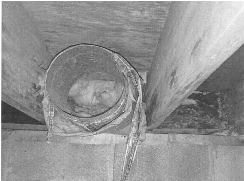
Photo No. 07 Location: Crawl space beneath building Description: Abandoned ductwork, typical.
