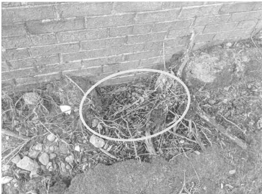
Photo No. 03 Location: Looking east at back of building. Description: Approximate location of crawl space vent beneath vegetation.
