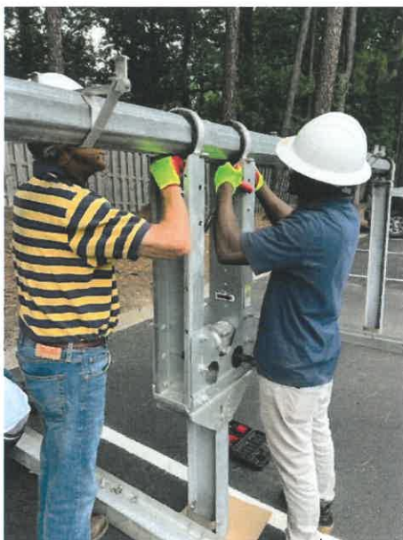
Instructor, Stuart Taylor, teaches a student the ins and outs of solar equipment and solar panel installation.
